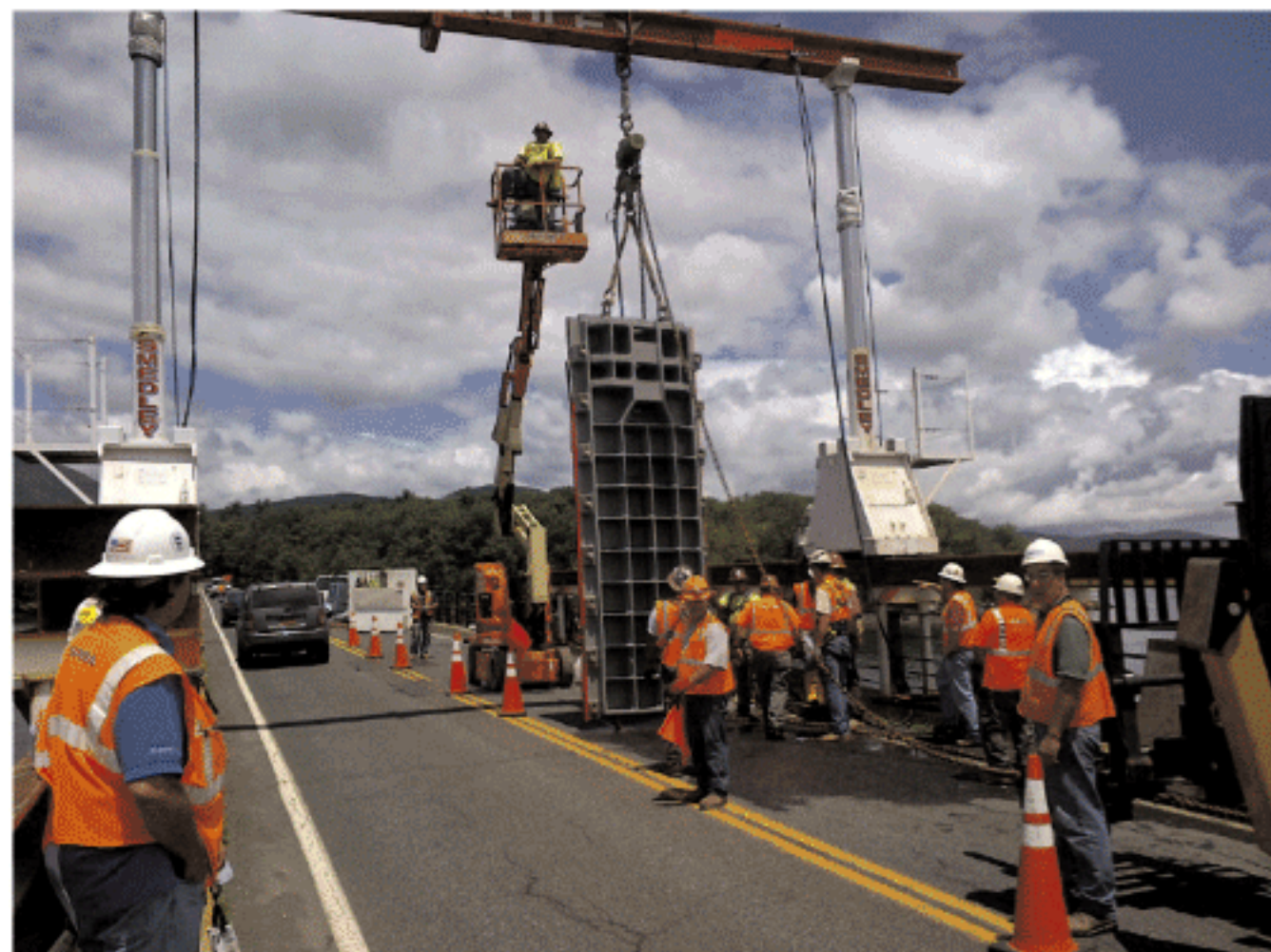
The four new gates are operated by individual motors, along with hand-crank backups, to prevent a single point of failure are installed.
