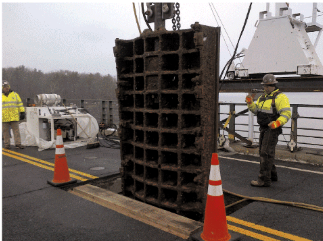
The original gates being lifted out of the chamber – the first time it had seen sunlight in more than a century!
