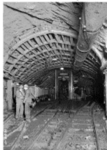
Hdq.d.1629, a photo of the Delaware Aqueduct water tunnel showing the steel supports and dump cars which remove the muck. Photo courtesy of the NYCDEP Archives.
