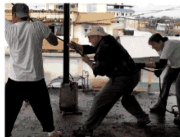
Pastor Bob and other team members hauling up piles of cement blocks to the 2nd floor.
